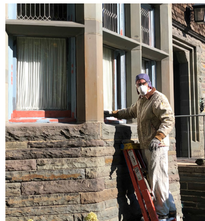
Terry Dunn, WSU staff, painting the and repairing the Freer House windows
